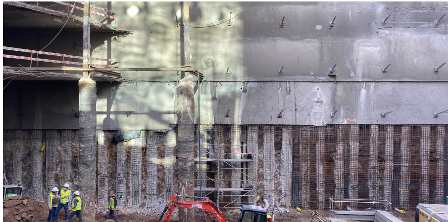
Figure 2 – Alignment D-E (northern area) – Pile curtain with a reinforced concrete wall and anchors
