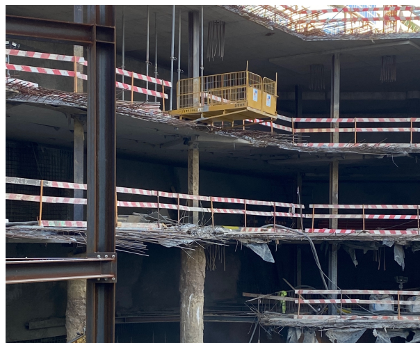
Figure 3 – Alignment B-C – Slab bands with HEB260 metal profiles working as temporary pillars
